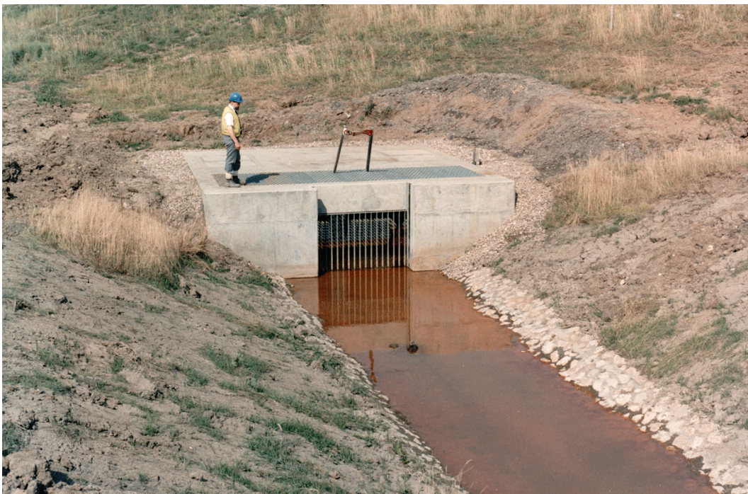
Plate 7.3 Outfall showing precipitation of ochre in channel at Carsington Dam
