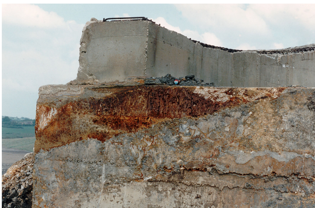
Plate 7.1 Concrete corrosion on spillway, Carsington Dam
