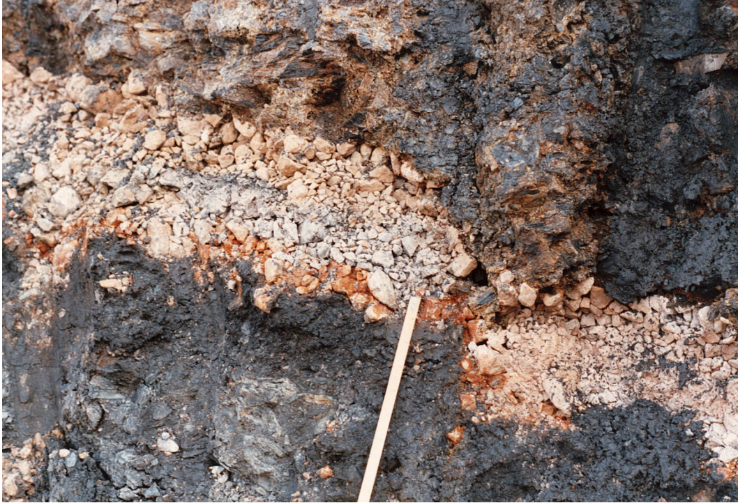
Plate 7.2 Chemical attack on limestone drainage blanket in acidic mudstone fill, Carsington Dam. Rupture surface to right of tape measure
